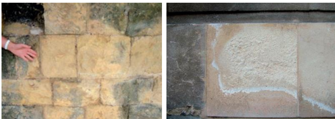
Figure 6: Typical salt deterioration and crystallisation to stonework of historic buildings (adapted from Viles, 2012)
