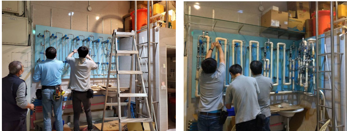
Figure 5 Assembly and water testing of insulated and non-insulated pipes of the same diameter and different pipe lengths
